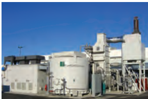
A smart grid and fuel cell were installed at Santa Rita Jail.
