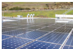
We have 13 large-scale solar installations.
