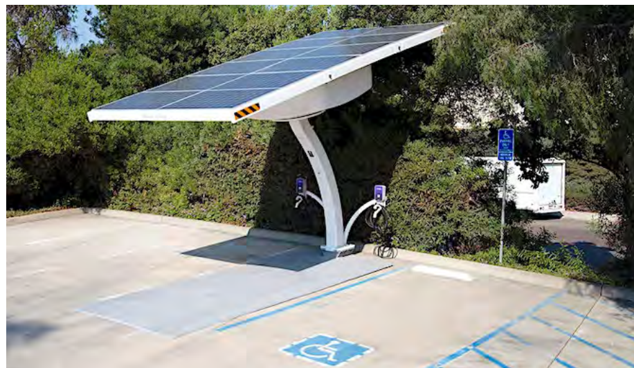
The EV Arc system is a portable system that can provide on-demand charging and back-up energy during a climate emergency.
