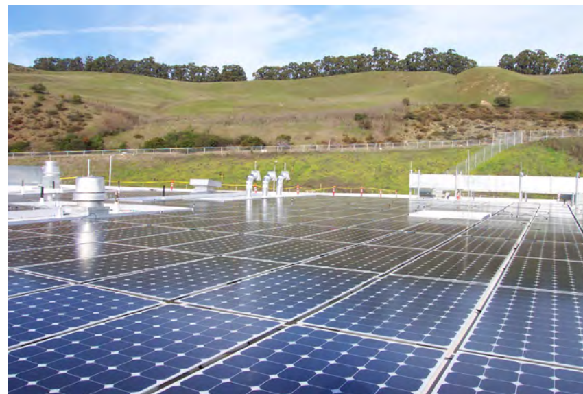
The Alameda County Juvenile Justice Center's roof hosts solar panels.
