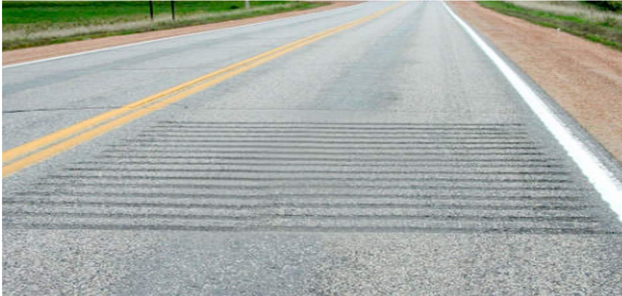
Figure 16 Transverse Rumble Strip
