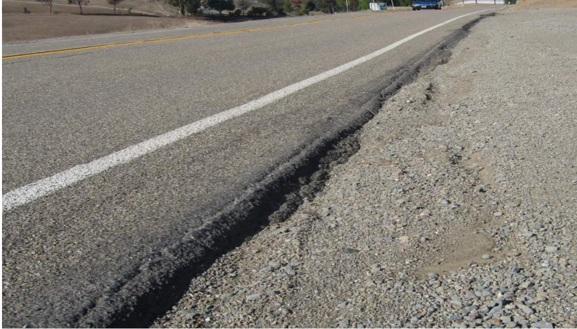
Figure 3 Shoulder drop-off with loose gravel
