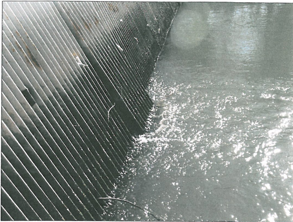
Upstream/Lakeside Trash Rack Displaced by Discharge Flow Also Areas of Coating Failure
