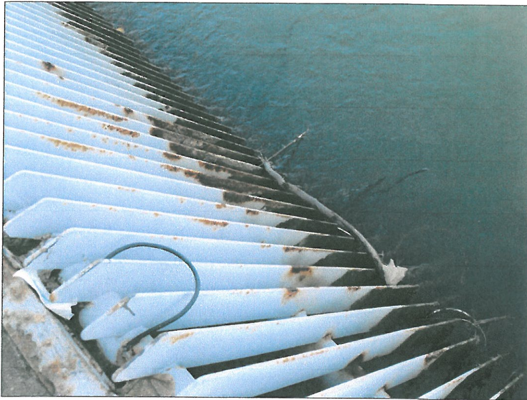
Upstream Trash Rack - Corrosion Example
