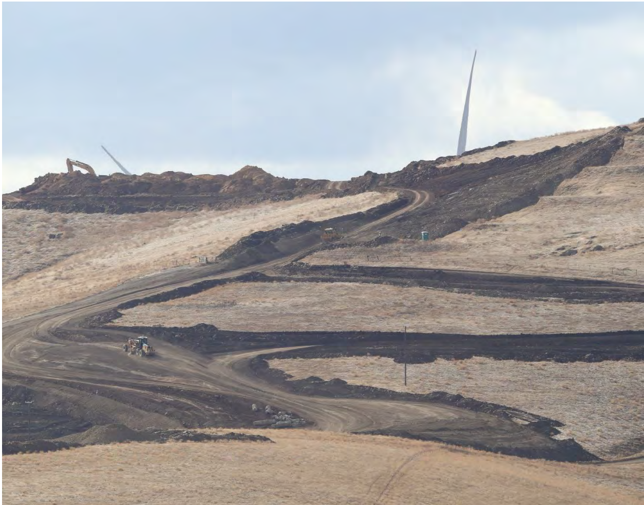
Photo 9. Construction grading for a repowered wind project destroyed every ground squirrel burrow complex encountered, which also diminished breeding opportunities for burrowing owls and forage for golden eagles, September 2019. This view includes only 2 wind turbine pads; the rest of the grading was for access roads.
