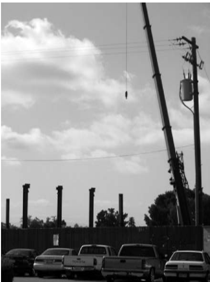
Performing Arts Center at Castro Valley High School under construction. School facilities such as this play a critical role in providing community facilities and defining Castro Valley's identity.
